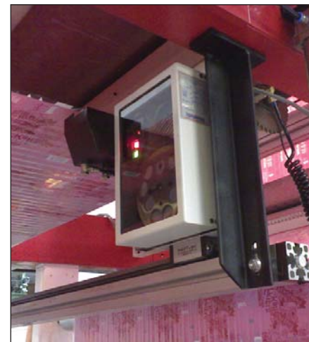
RTIS 2 unit mounted upside-down, firing up onto laminate.
